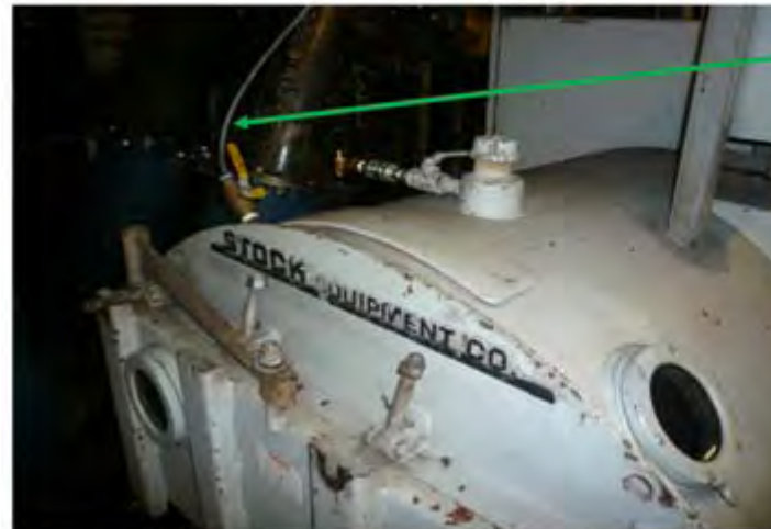
Injection point to one feeder
